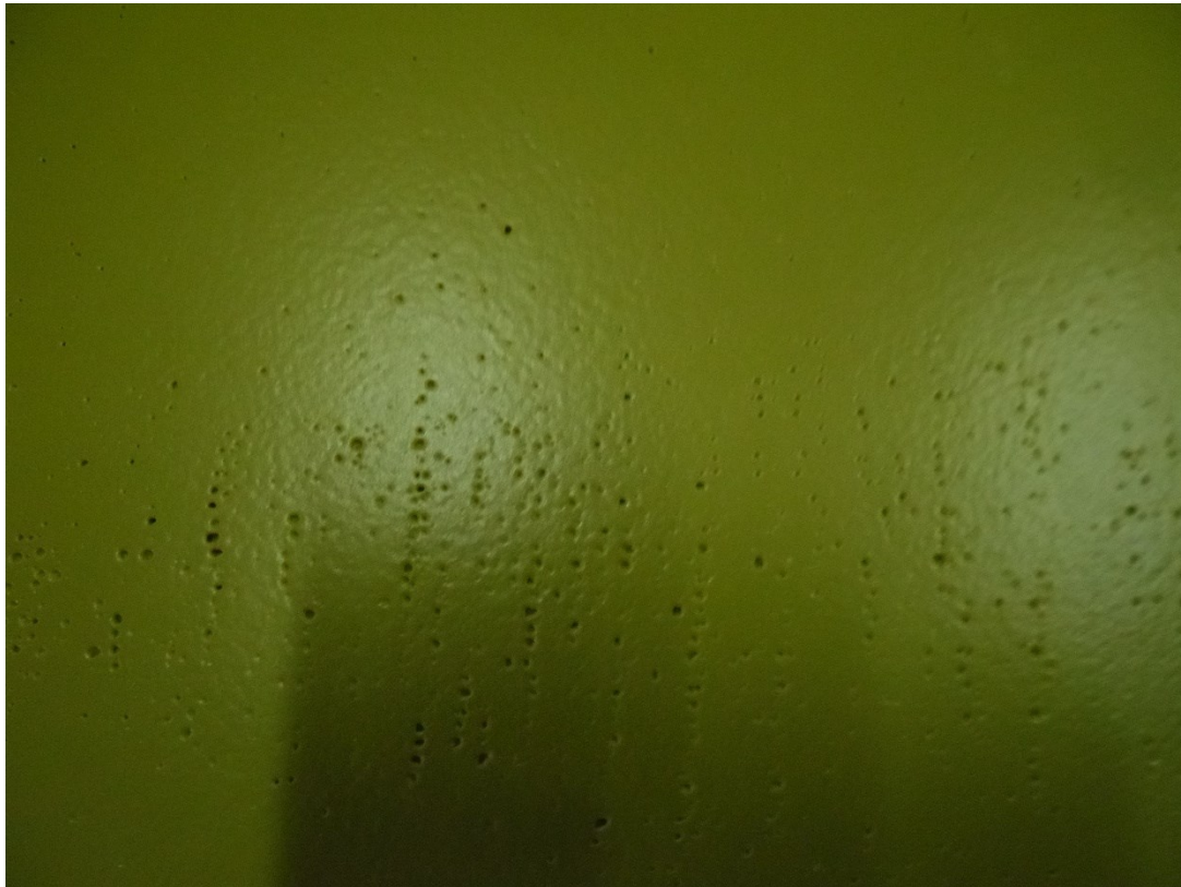
Figure 1 Too many pinholes
